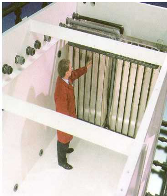
Figure 9b. Immersed Microfiltration Membrane Installation
