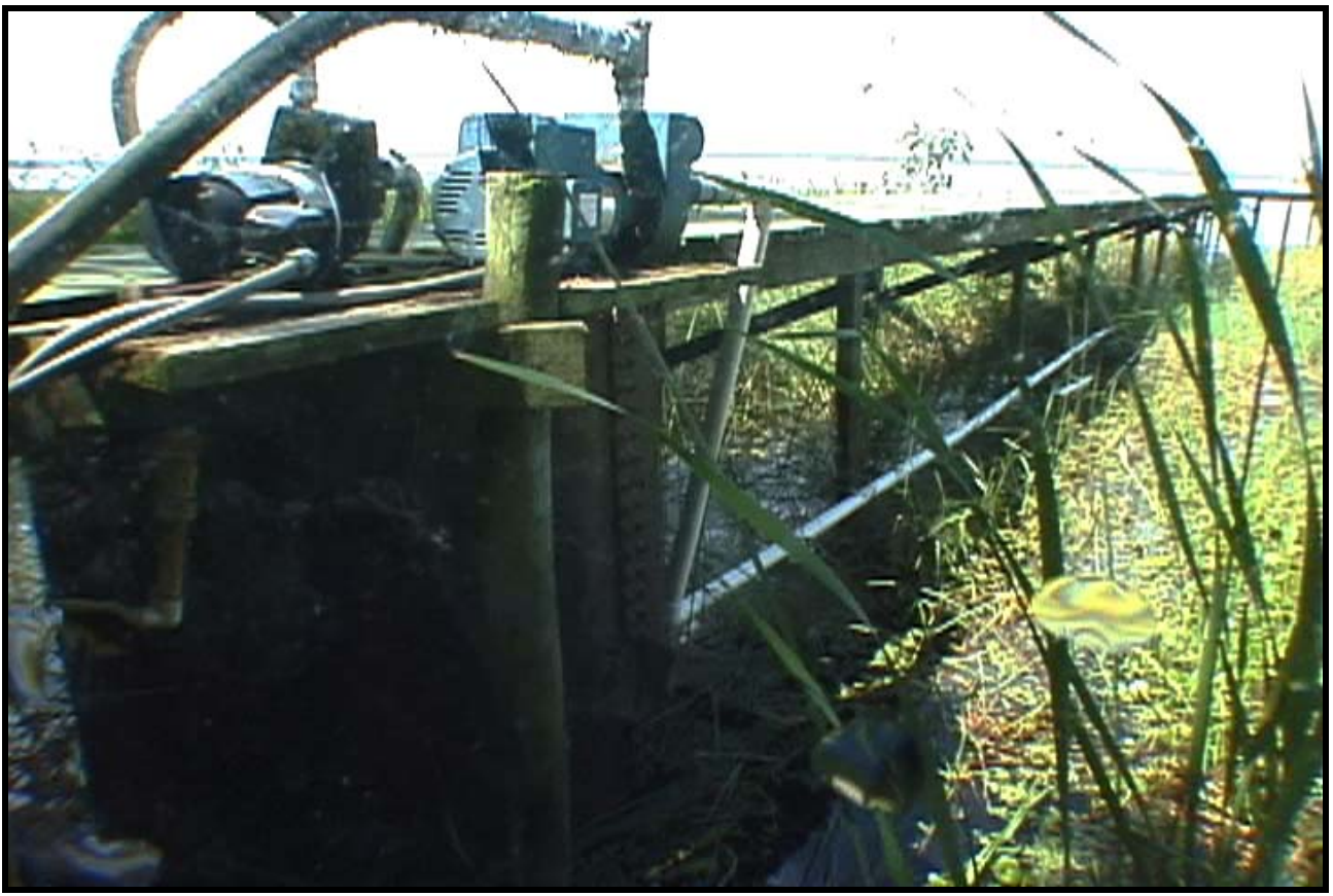
Figure 11. Video still of Lake Harris Dock Spring, Lake County, Florida. Spring is encased in large diameter steel casing below pumps on right side of picture.
